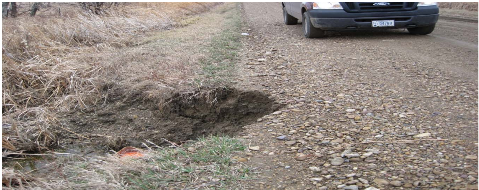
Deteriorating road conditions on the Fort Peck Reservation.
